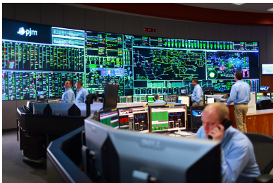
Control Room calls [10]
